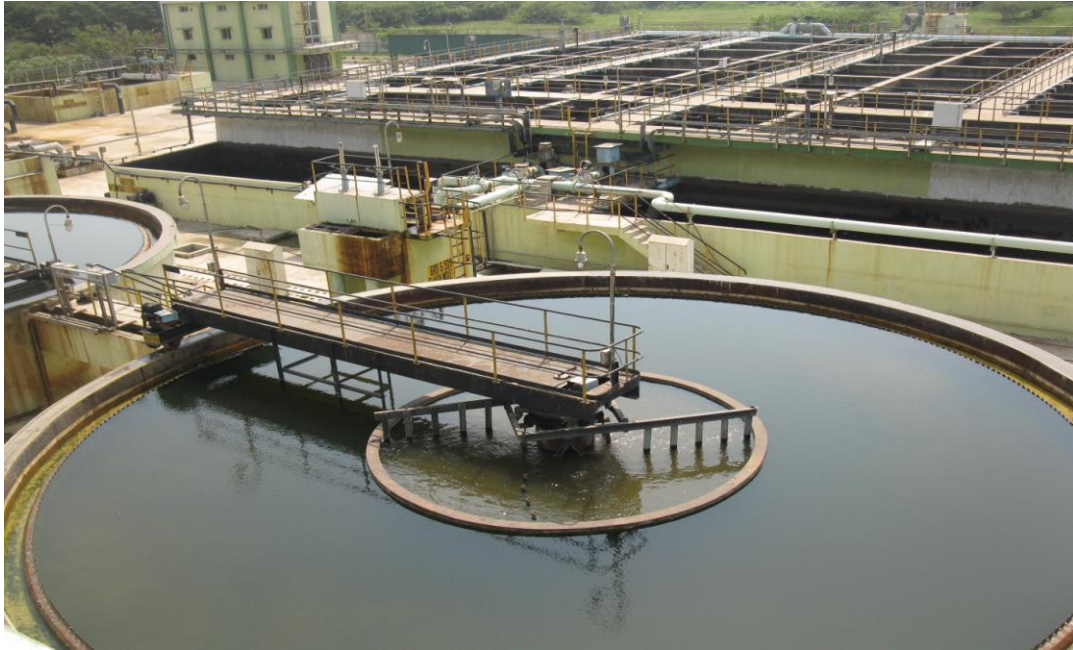
Sewage Reclamation Plant -2 (SRP-2)
