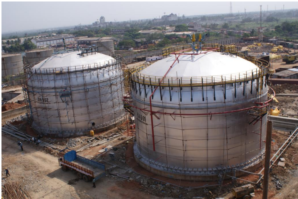
Dome Roof Tanks with Nitrogen Blanketing
